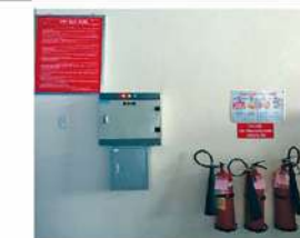
Example fire protection equipment provided for the storehouse
